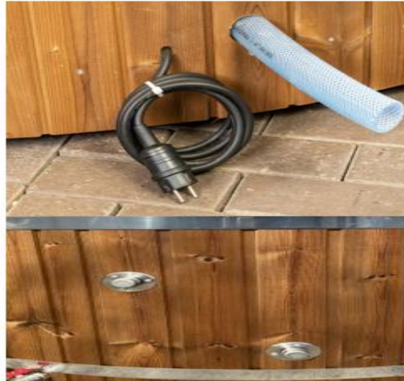
Figure 27: 230 V earthed plug for hot tub (to the right: Preparatory work for the sand filter unit (water return pipe to the sand filter unit))
